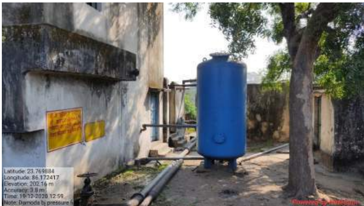
FILTER PLANT IN THE MINE AREA
