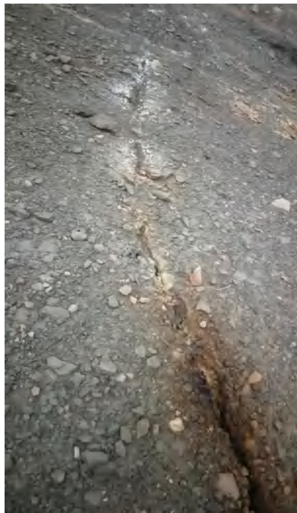
Figure 20: Fume cracks in the Bhulanbarari area.
